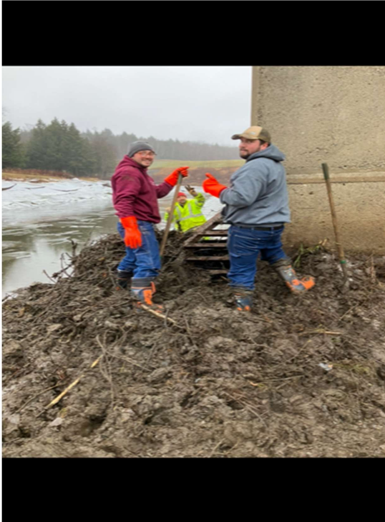
Water Dept Crew – Beaver Dam Dig-out Photo by Joe Gaudiana, Chief Operator
